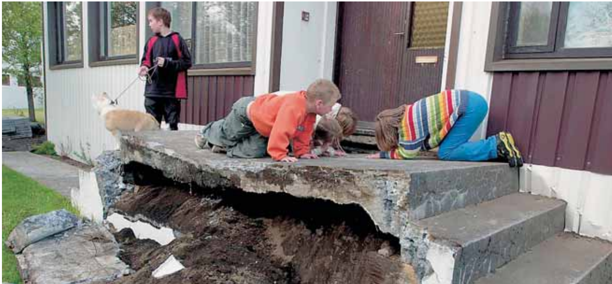
Children, looking at a damage caused by the South-Iceland earthquakes in the year 2000
