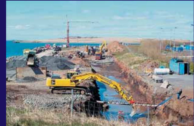
Installation of a Ø1,4 m main waste water pipe in Leirvogur, Reykjavík
