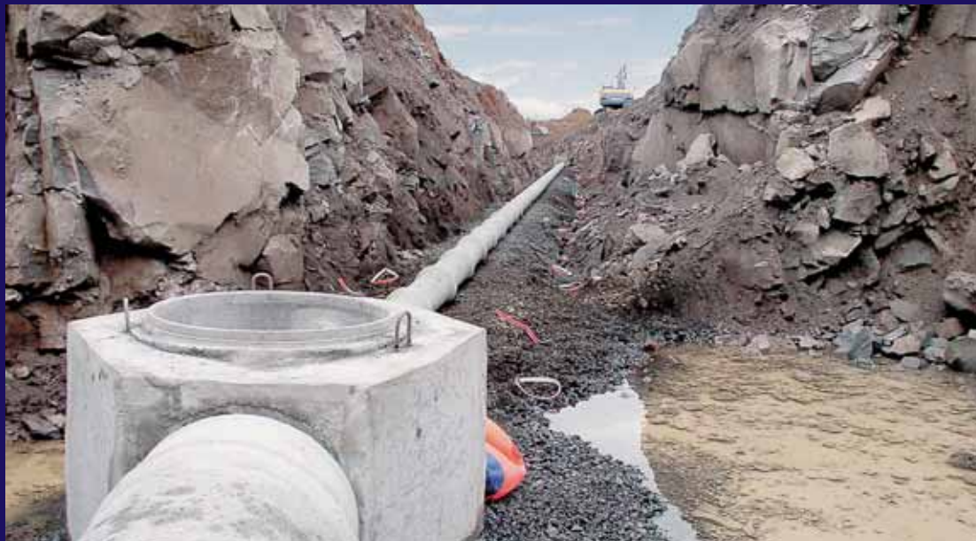
Wastewater collection system in Norðlingaholt
