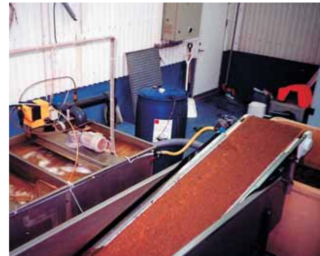
Waste water treatment unit for an industrial company
