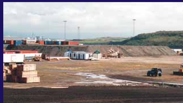
Preloading of a building site on a reclaimed land at Vogabakki, Sundahöfn Photo: Almenna
