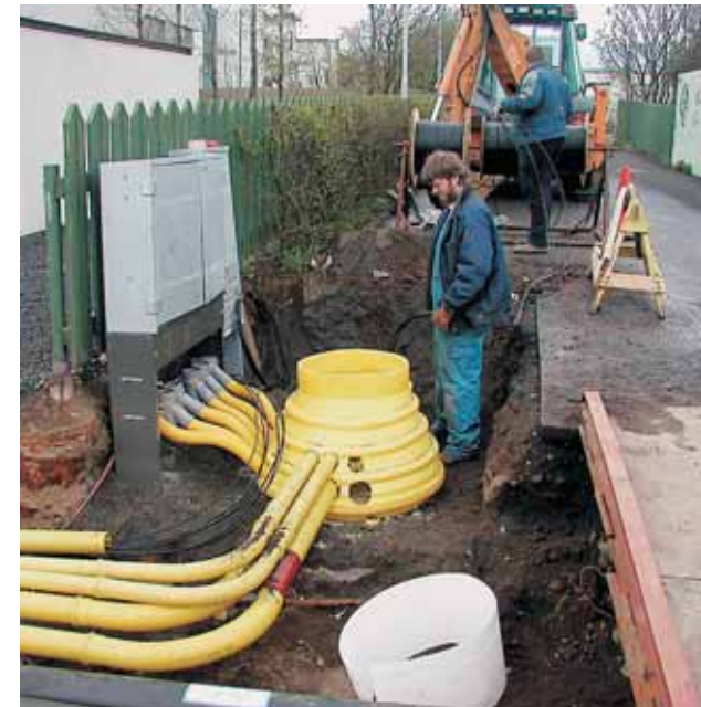
Renewal of municipal distribution systems in the older districts of Reykjavik Photo: Almenna
