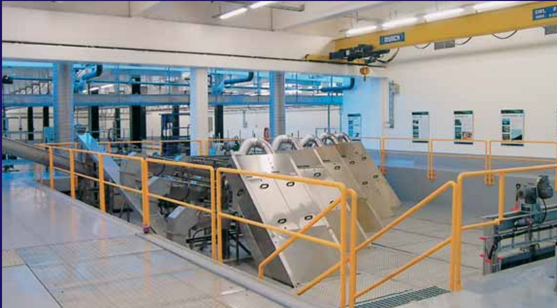
Step screens in the waste water treatment plant at Klettagarðar, Reykjavík
